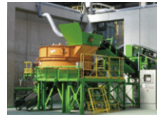
Manufacturing Facility for Cement Raw Material
