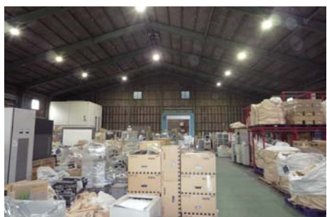
LED lighting system on the high ceiling at Saitama RC
