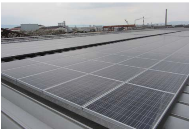
Photovoltaic module (Amagasaki Plant at Hanshin Business Office)
