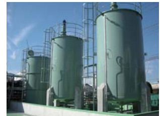
Waste Oil and Product Storage Tanks
