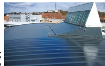
Photovoltaic energy generation roof (Techno-Center)
