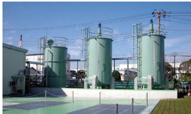
Waste Oil and Product Storage Tanks
